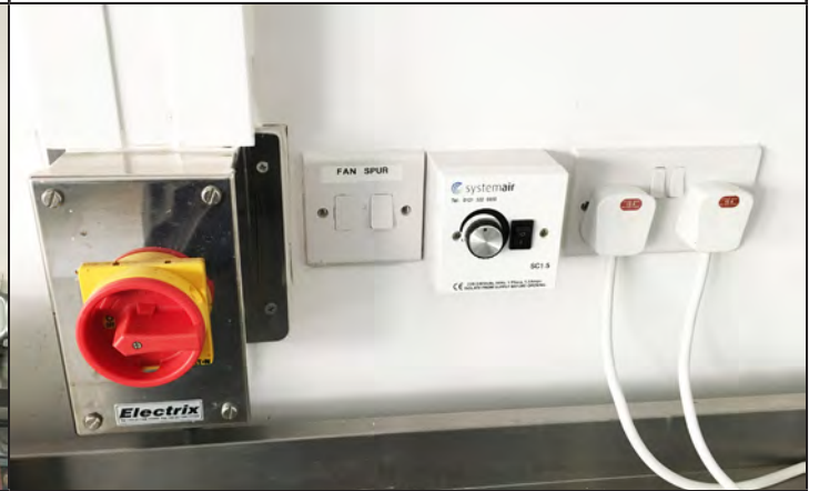
Electrical Isolater Oven extractor controls
