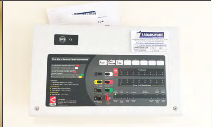
Fire Alarm Panel
