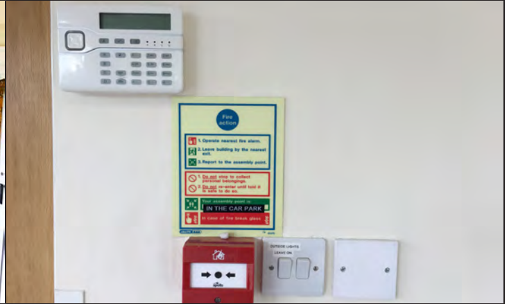
Entrance – Fire Alarm including Security Alarm Panel & signage
