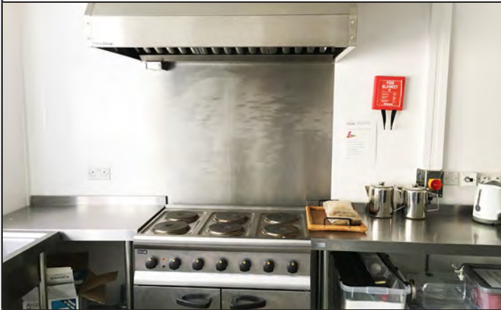
Industrial Oven, Fire Blanket, Kettles
