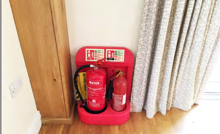
Fire Equipment - LH Push-Bar Exit South Elevation
