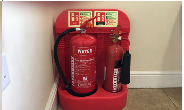
Foyer Fire Equipment
