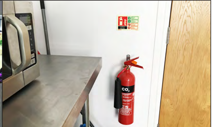
Microwave & CO2 Extinguisher
