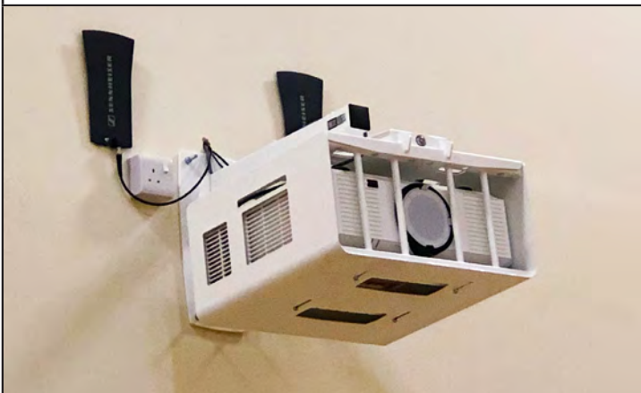
Projector Mounted on North side internal wall
